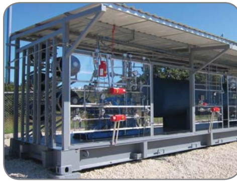
H2 Fuel Station
